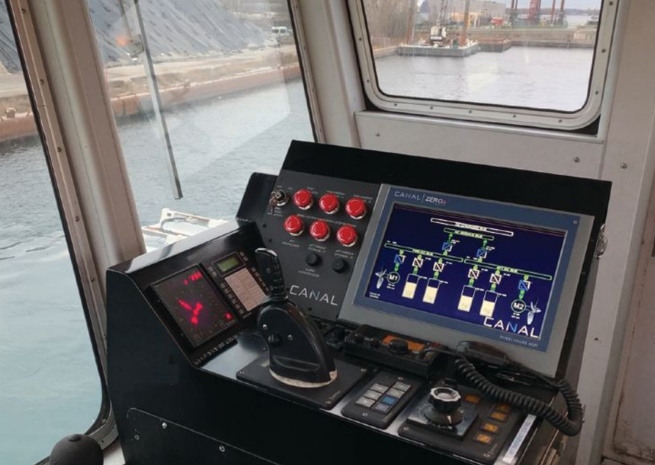
(Left) Onboard ferry controls used by the operator. The digital display shown here depicts the electrical system. (Below) Marilyn Bell is now a fully electric ferry with resulting zero emissions and lower operating noise.
