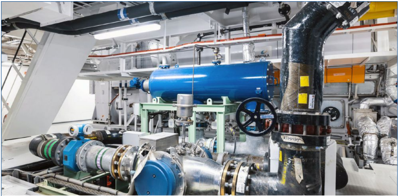
Wärtsilä Water and Waste's Aquarius ballast water management system on board MS Viking Glory.
